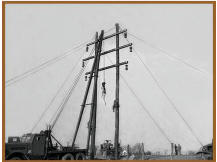
Early cooperative employees work on Kentucky's transmission system, helping expand reliable electric service to rural communities. Investments like this laid the foundation for the communities and economy we serve today. Photo: EKPC Archives
